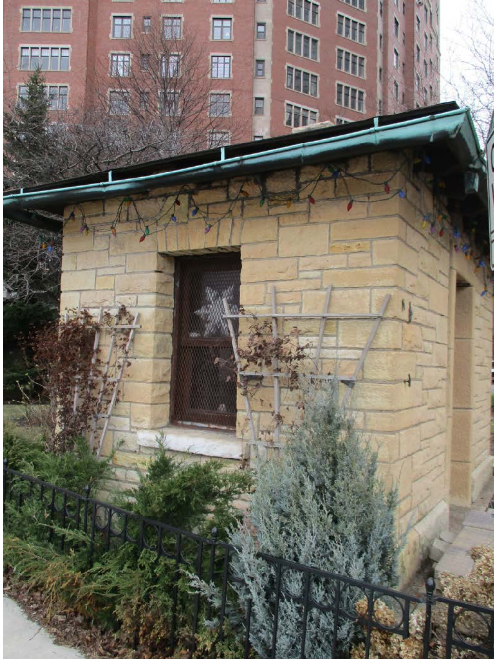
Park Structure, view looking southwest from N. Lake Shore Drive toward East façade
