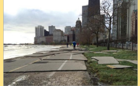
Lakefront Trail pavement damage (via Twitter)
