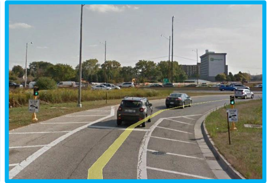
Ramp Meter Signal
